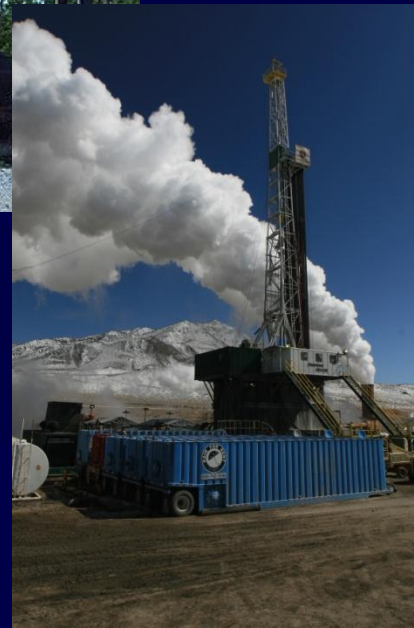
Geothermal well 2000 gpm
